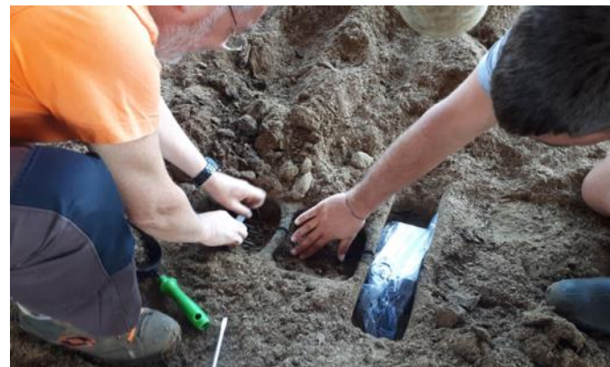
Litter temperature and humidity sensor installation
